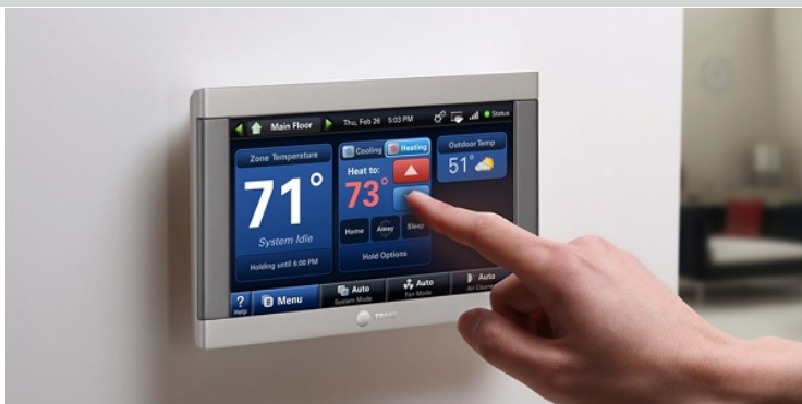
Figure 28: This smart thermostat allows attackers to gain remote access, and breach the rest of the network.
