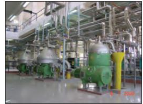
A piping network in an industrial facility.
