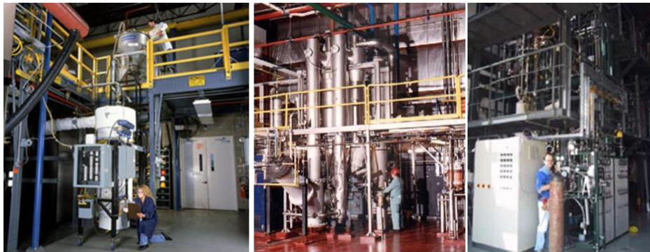
Biomass Pyrolysis Pilot Plant
