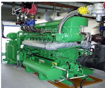
CHP Biogas ICE - 600 kW
