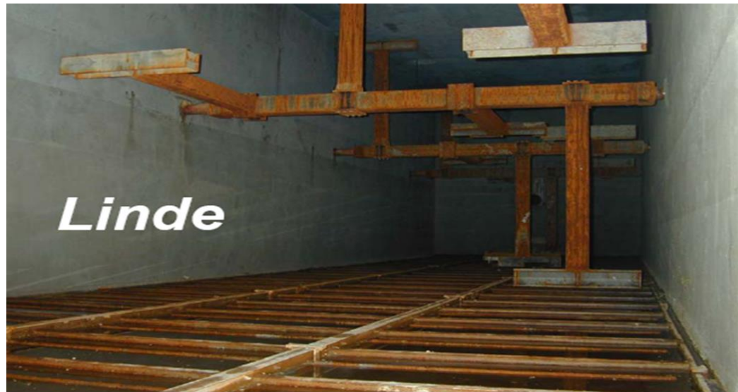
Plug Flow Digesters
